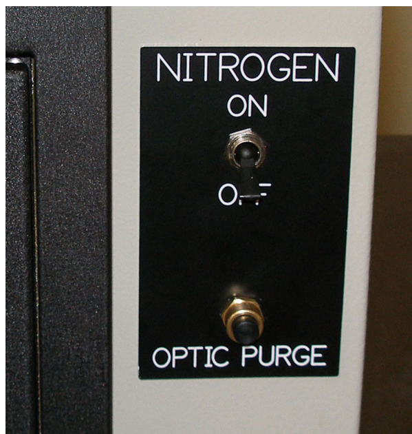
Figure 2-19, Sulfur Optic Control Panel
